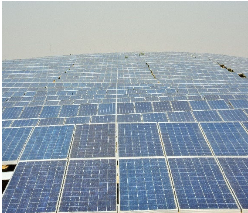
150 MWp Ground Mount Solar Project, Rajasthan
