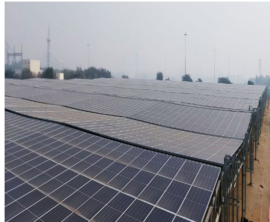
20 MW Solar Carport project, Haryana
